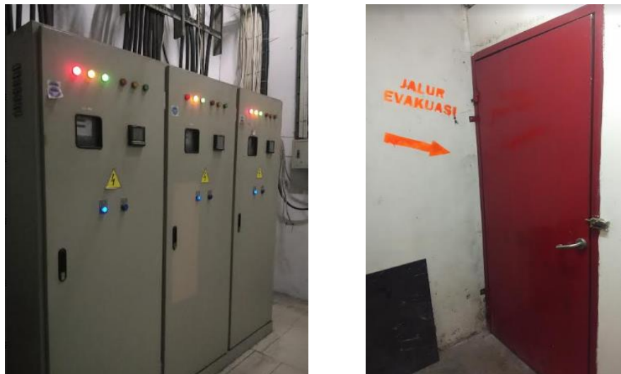
Figure 1. Electrical panels at JCM and The Rich Hotel and Mall Evacuation Routes
