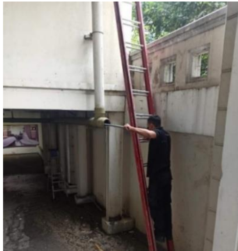
Figure 2. Hotel Drainage Leaks
